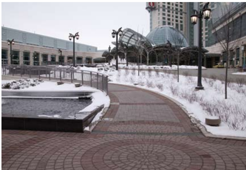
REHAU SIM system clears vehicle and pedestrian pathways around the Fallsview Casino Resort in Ontario.
